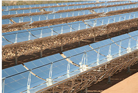
Figure 2: At APS's Saguaro Generating Station, six rows of 15-foot-high mirrors generate electricity by heating oil to drive steam turbines. (Photo by Arizona Public Service Company)
